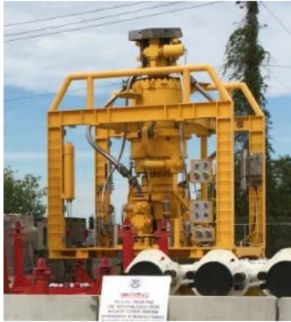
Figura 2.18 – Blowout Preventer (BOP) [21]
